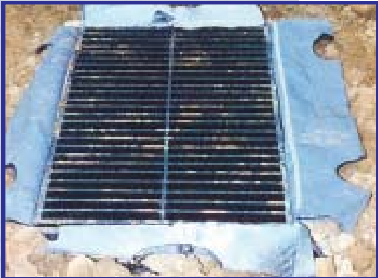
installed Siltsack held in place by grate.
