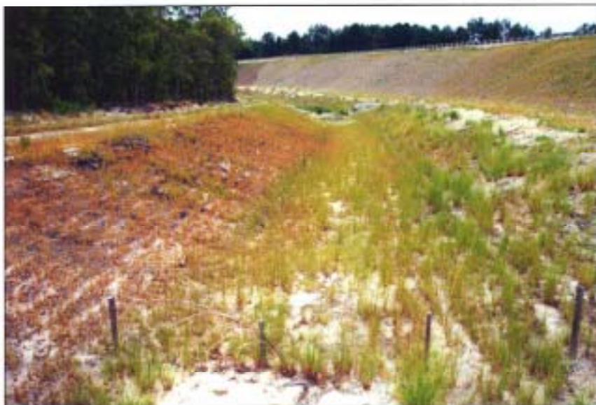
Vegetation begins to grow through the Pyramat® matrix just a few weeks after installation.
