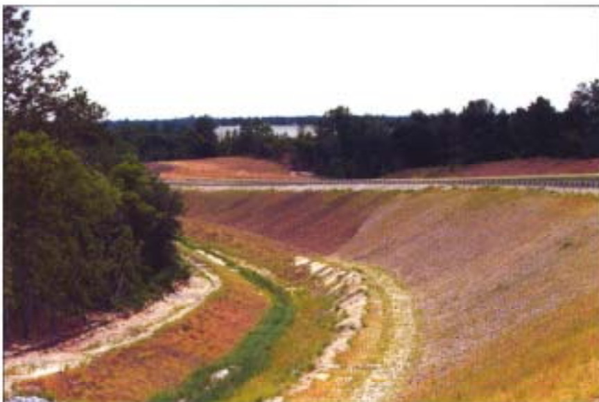
Pyramat® was used to line two channels that totaled more than 3,000 feet in length.
