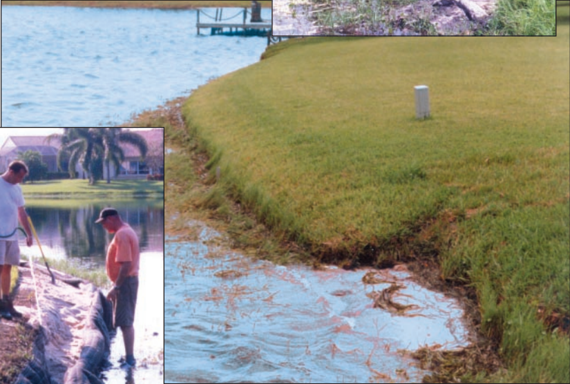
Landlok TRM 1061B was placed, filled with sand, wrapped as illustrated in the detail and sodded. The result is a natural looking residential shoreline.
